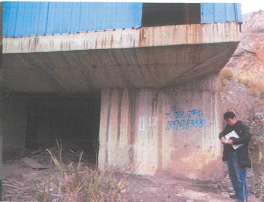
17-2 厂房外破碎机料仓
